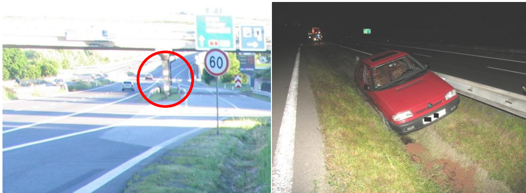
Fig. 7. High risk location 1– missing protection of concrete construction of the bridge
