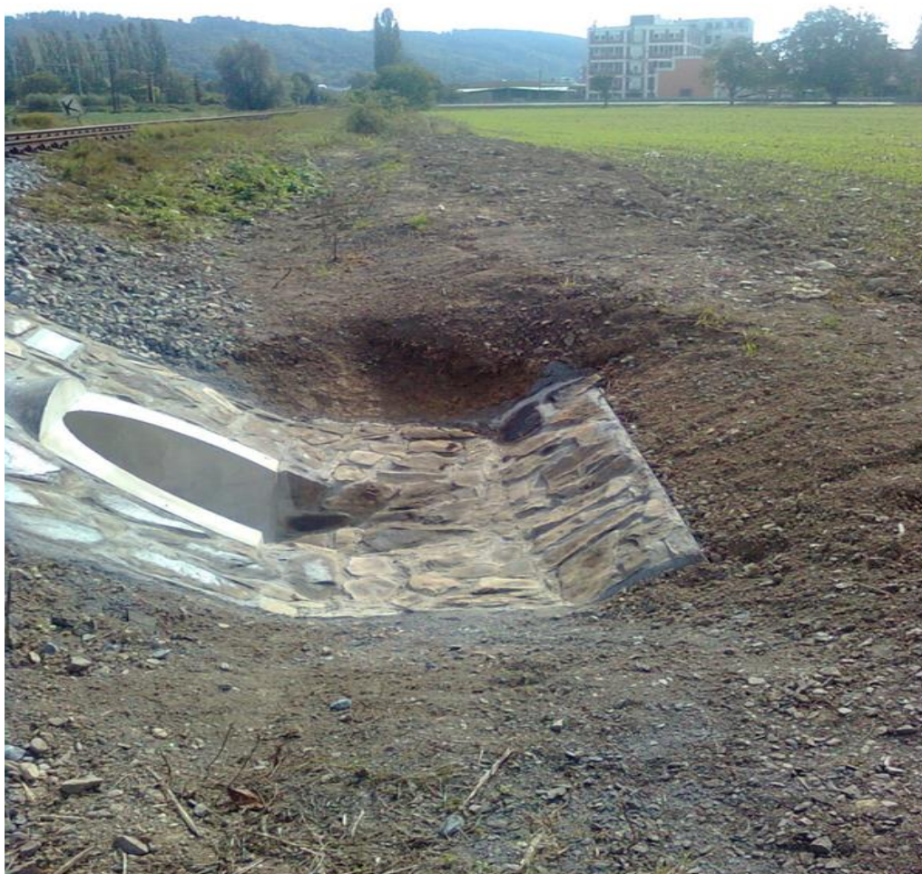
Figure 3: Implementation of the culvert under the railway apparently systematic and conservative solutions investments managers of highway construction. The construction does not fulfil the purpose for which it is designed
