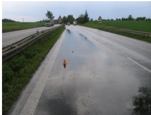
Fig. 10. High risk location 3 – detail of condition of the road surface
